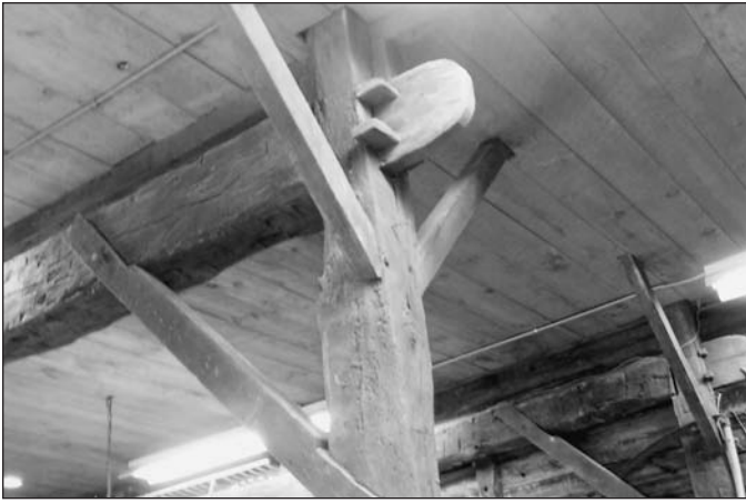
Photo 7. An interior photograph of the Yeoman-Abma barn. Prominent in this view is a 13" anchorbeam tenon extension with double wedges. The purlin braces that extend below the anchorbeam are quite typical of Bergen County barns. Note the H-frame braces with lapped half-dovetail joinery.
