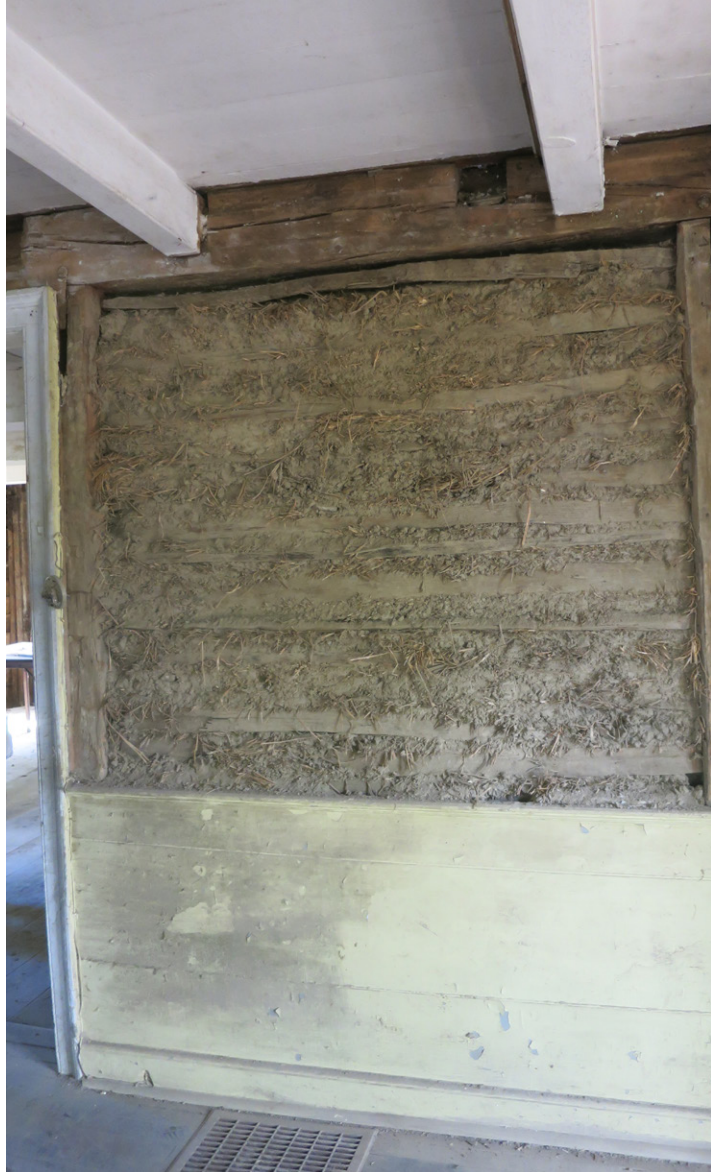
Mud-packed substrate in wall at 246 Spring Lake Rd., Upper Red Hook (October)
