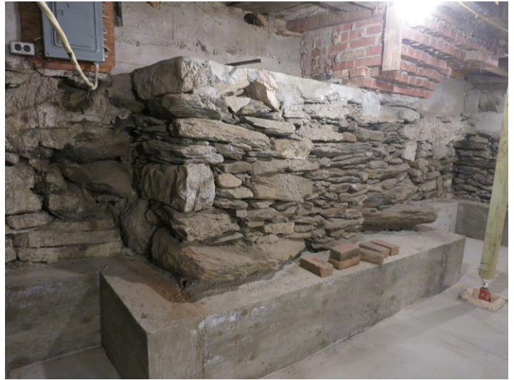
Fig.8: View of west end of basement showing stone base for chimney replacing original jambless hearth. Brick chimney is a later addition when room above was divided. Photo by W. R. Wheeler, 2019.
