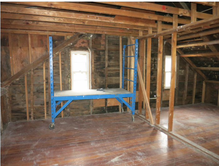
Fig.9 View of east end of attic showing where rear portion of roof was raised; original front rafters visible on right. Photo by W. R. Wheeler, 2019.
