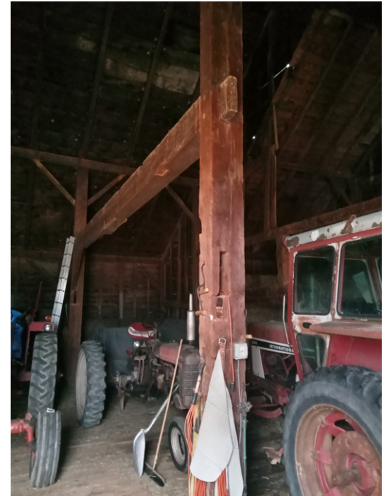
Fig. 4: Bent three, with mortises indicating a second anchorbeam. Photo by Ted Hilscher.
