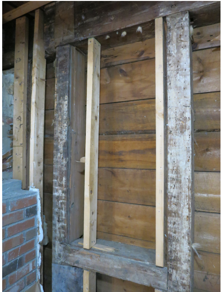
Fig.6: Detail of window frame on west wall. Photo by W. R. Wheeler, 2019.
