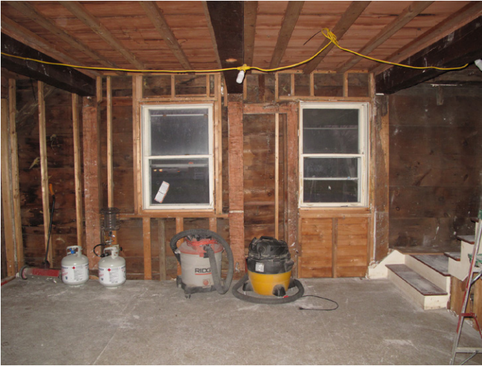
Fig.4: View looking south on east side of house showing remains of wall framing for window and door (see Fig. 5). Photo by N. Larson, 2019.
