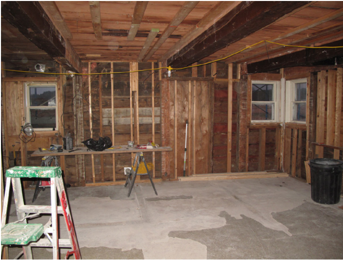
Fig.7: View looking northeast showing ceiling beams with original paint, hacking for addition of lath and plaster, and evidence for later ceiling with stained beams and gypsum board ceiling covering floorboards. Photo by N. Larson, 2019.
