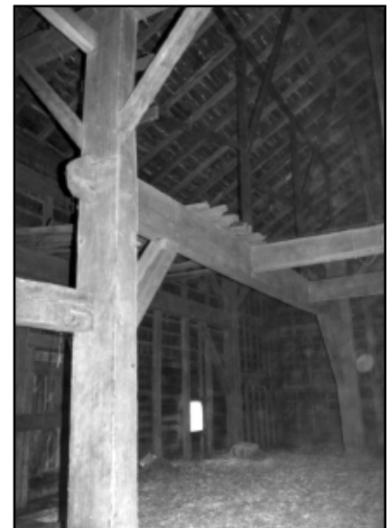
Photo 9. The Schenck barn, view of first inner H-bent. Two horizontal beams at the right side of the photo joined to the middle anchor-beam, thought to have been about 26 inches in height at its midpoint (Photo by Gail Hunton).
