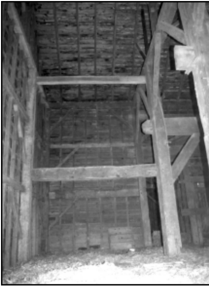
Photo 10. One of the end bays in the Schenck barn. Note the very large lower transverse end bay tie that may have been original to the three-aisle barn. The tie was 13 inches in height (Photo by Gail Hunton).
