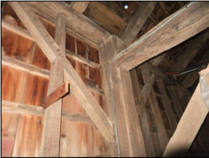
Photo 16. View of the Dutch-Anglo barn on Vanderburg Road in Marlboro with heightened eave-wall H-bent post that rises above the level of the "Dutch" purlin plate seen at the upper right. This feature proves that the barn was originally built as a Dutch-Anglo barn. Note horizontal slats where exterior wood shakes were originally nailed (Photo by Greg Huber).
