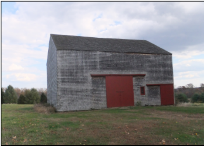
Photo 15. The Williamson-Sickles Dutch-Anglo barn on School Road East in Colt's Neck has three "Dutch" bays in the middle bay of this three-bay barn. This barn was likely built c. 1830 (Photo by Greg Huber).
