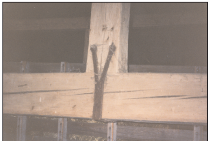
Photo 14. Detail of interior of double-decker barn at the Wickersham farm in Chester County, Pennsylvania, dated 1809. Note the forked metal support that connects the vertical king post to the swing-beam, which spans more than forty feet.
