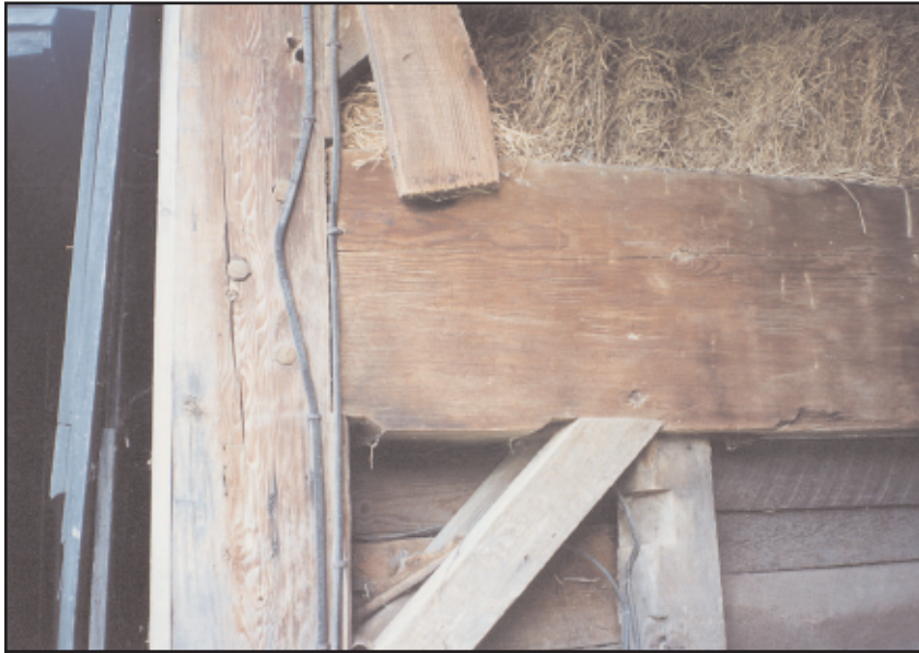
Photo 13. View of double end braces that join the swing-beam of the Barber barn to its side-wall posts. Note the three pegs at union of beam to post and use of square shouldering.
