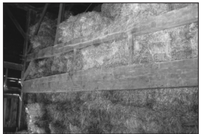
Photo 1. Interior view of bent showing a substantial swing-beam in a ground barn in Bethlehem Township, Warren County, New Jersey. The bent that flanks the wagon bay also has an upper tie beam and the side-wall post extension above the upper tie is quite long. (All photos by the author unless indicated otherwise).
