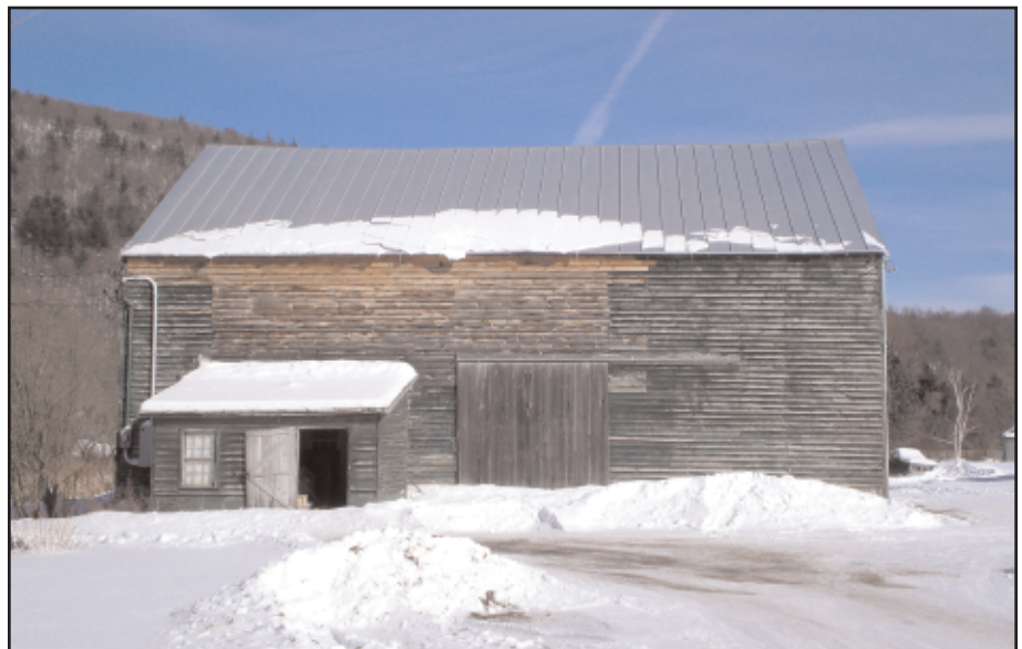
Photo 10. Exterior view of Barber swing-beam barn near Schoharie, New York with its horizontal siding and side-wall wagon entry (Photo by Grace Barber).
