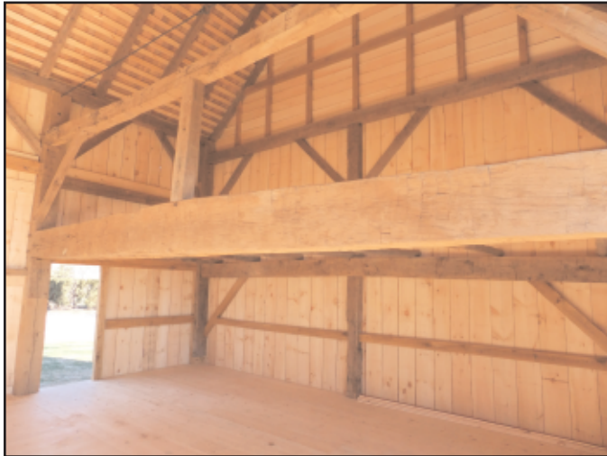
Photo 5. The 1'-7 1 / 2 " high swing-beam of the same barn, which measures 36 by 26 feet overall.
