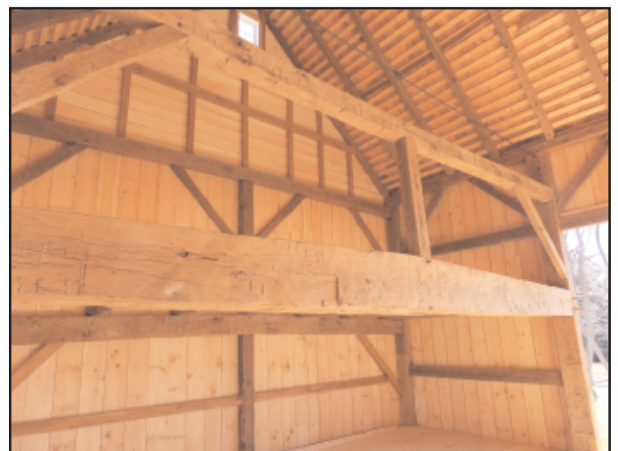
Photo 4. Interior view of the side-wall entry ground barn in Cranbury, Middlesex County, New Jersey, showing the expansive upper area of the end bay beyond the swing-beam.
