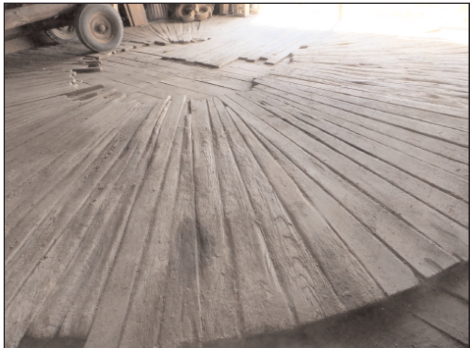
Photo 6. View of circular arrangement of tapered planks in a shed attached to a Pennsylvania Standard fore-bay barn in Lehigh County, Pennsylvania.
