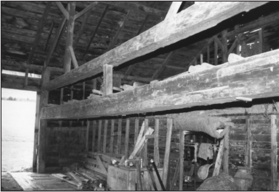
Photo 11. Interior view of bent includes a swing-beam in a ground barn in Schoharie County on Route 443 in New York. This bent flanks a wagon bay and has an upper tie beam; the side-wall post extension above the upper tie is quite short.
