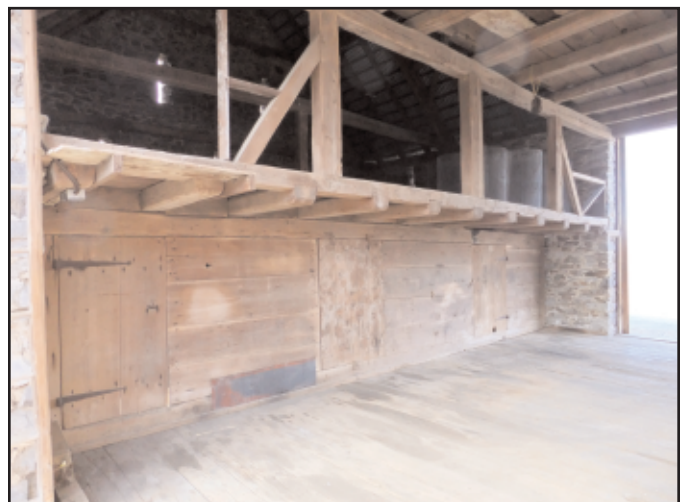
Photo 8. Interior cantilevered beams support a transverse beam in this circa 1785 barn in the Oley Valley, Berks County, Pennsylvania, which may have functioned as a swing-beam.
