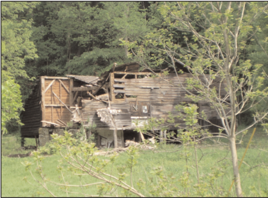
Photo 2. The LeFevre barn with roof collapsed, May 2009. The side walls remain mostly intact but the south end wall has fallen. Trees have been encroaching on the barn for a number of years.
