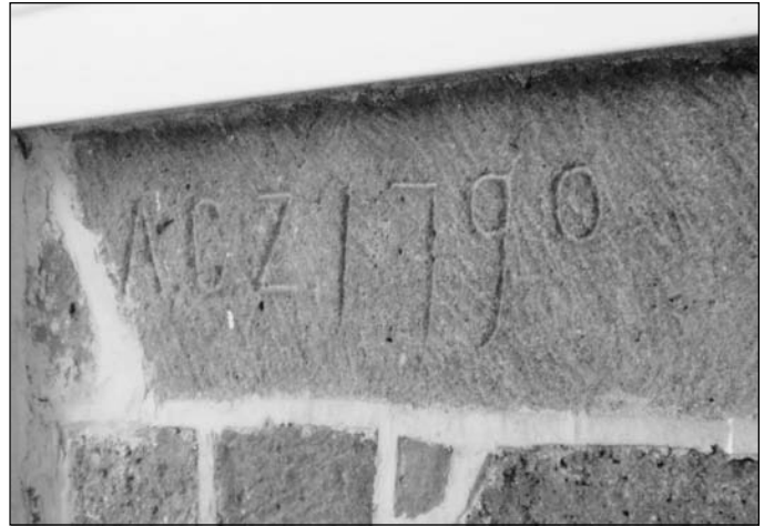
Photo 6. Detail showing initials and date carved in stone: ACZ 1790 on the Zabriskie barn. This date is probably not the date of construction, which is likely earlier by a decade or two or more.
