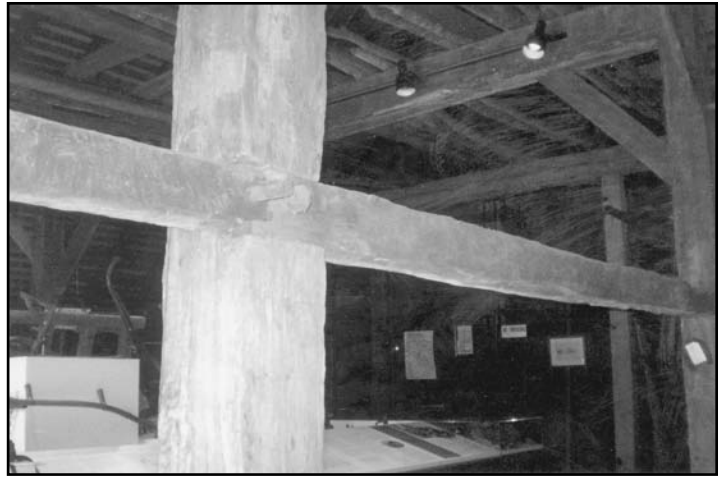
Photo 1. Interior of the c.1760 (dendrodated) Wortendyke three-aisle barn has longitudinal struts lapped onto widely slotted H-frame posts. These lapped struts are often seen in Bergen County and Rockland County barns and are considered a regionalism.
