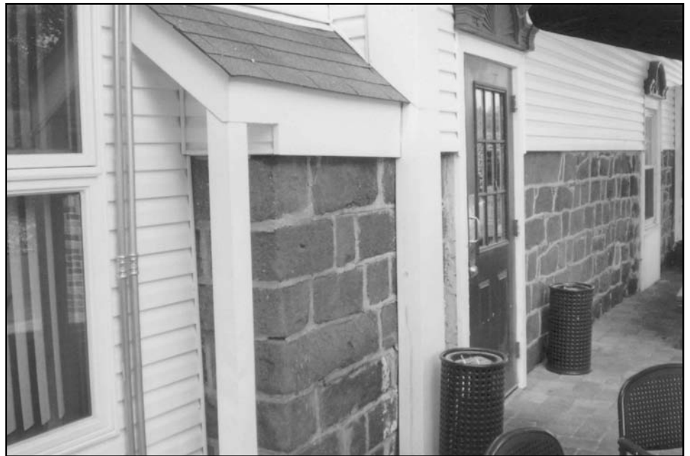
Photo 5. A detail of a side wall of the Zabriskie barn, the only known extant Dutch barn with side walls of stone construction. This native stone is often the same type seen in innumerable Dutch stone houses in Bergen County.
