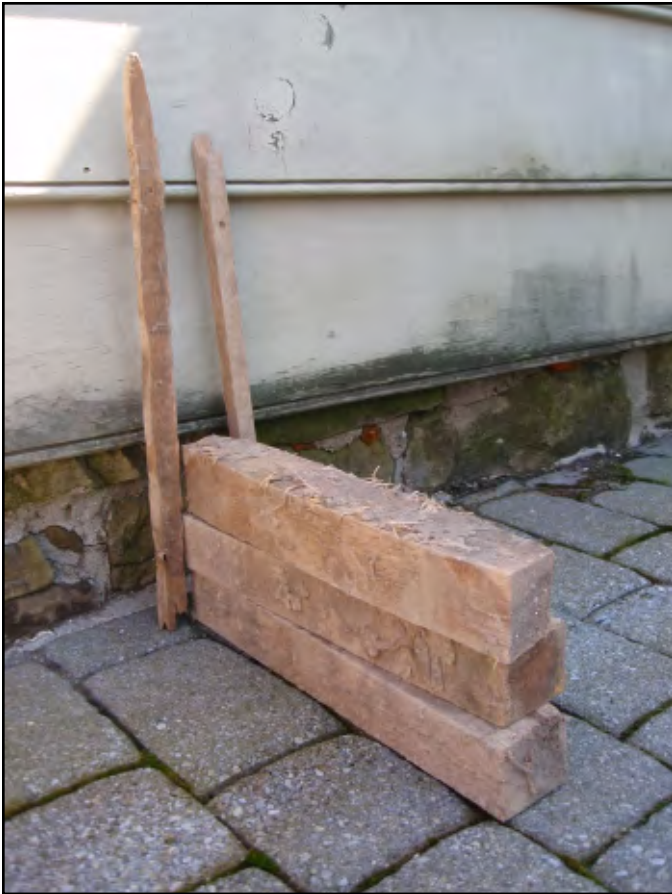
Photo 4. Some of the components of the wall infill. Mud and grass was packed around each of the horizontals which spanned between the bent posts of the house.
